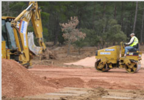
Levelling the land in preparation for the next temporary ITER building. Click on the picture for a high-resolution image.
